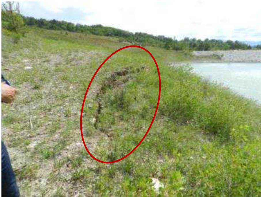
Figure 9 : Fissuration (Source : INRAE)
